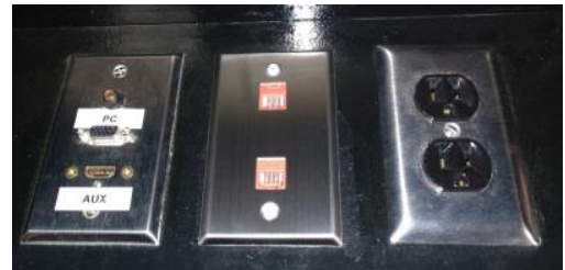
Room 122 Wall Plates (on top of entertainment center)
